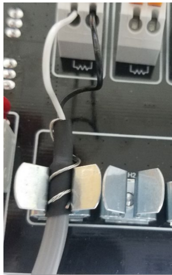
Figure 18: BOM cable inserted into 360° shield connection
