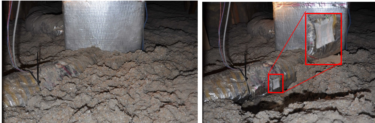
Figure 2. Photos of buried duct (left) and exposed moisture sensing strip (highlighted, right)
