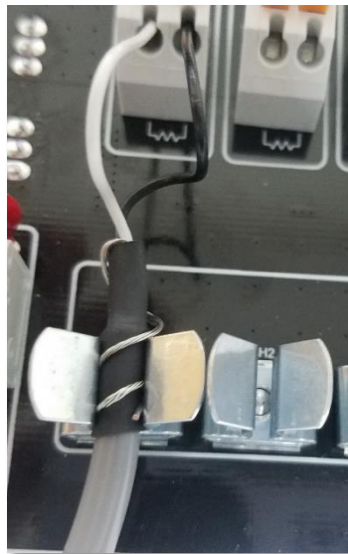
Figure 18: BOM cable inserted into 360° shield connection
